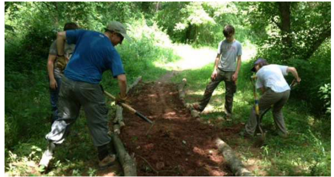
"Turnpiking" a trail – building up low, wet areas to ensure proper water drainage
